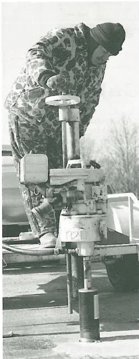
Orville Wiggins, District One Lab Technician, removes a core sample for testing.
